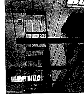
STEEL CABLE GUARDRAIL
